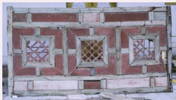
Panel from one of the rawashin from the Governor's Residence, during conservation.
