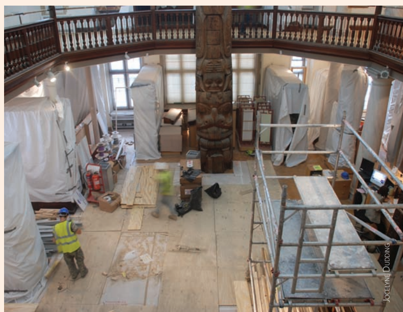
Upstairs during the Museum building work, with the totem pole and other very large items shrouded within the scaffolding.
